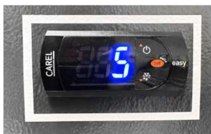
Electronic control panel
